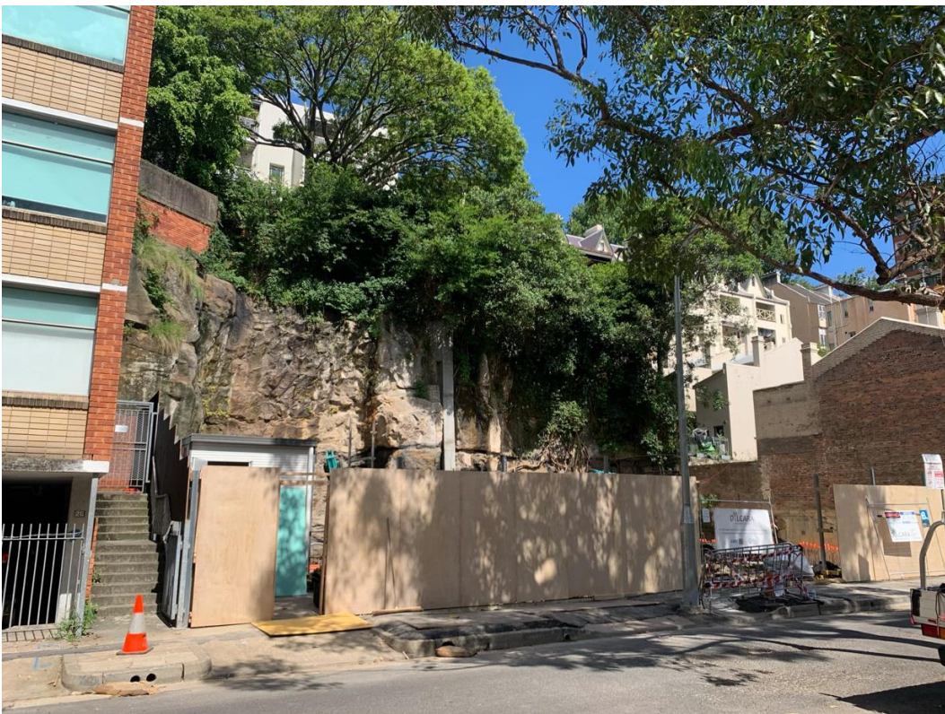
Figure 6: Adjoining site under construction to the southwest at 30A-34 Brougham Street, viewed from Brougham Street
